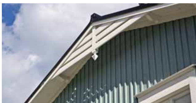
• Profiled support brackets and moderate gingerbread work embellish the gable ends. The siding of fresh-cut timber dried quickly and could be painted in a beautiful bluish-green colour.
