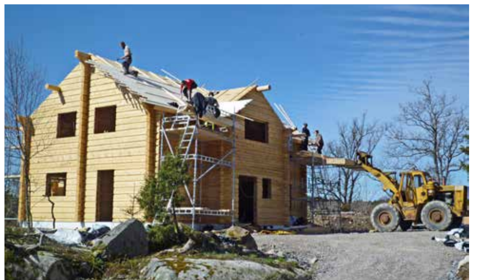
• During spring 2012, the timber frame was erected and the house got its roof of self-made T & G boards.
