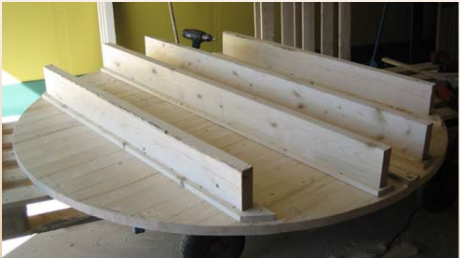
The fixing boards and the bottom joists are screwed together into T-beams, which then are screwed to the bottom. The ends touch the 20 mm line.
