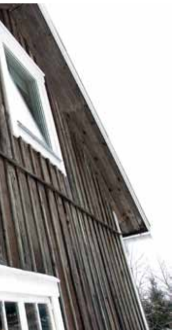
• The panelling was treated with copper and then put to lie outdoors for a year, just to get the right shade of grey.
